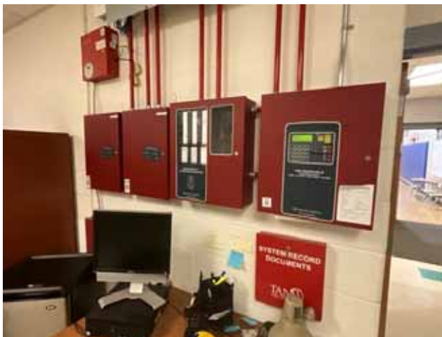
23 - FIRE ALARM PANEL
